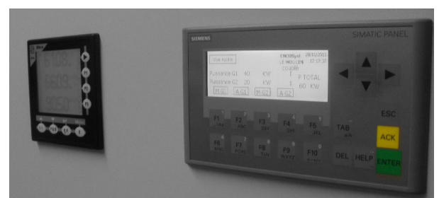
Panel de control local
